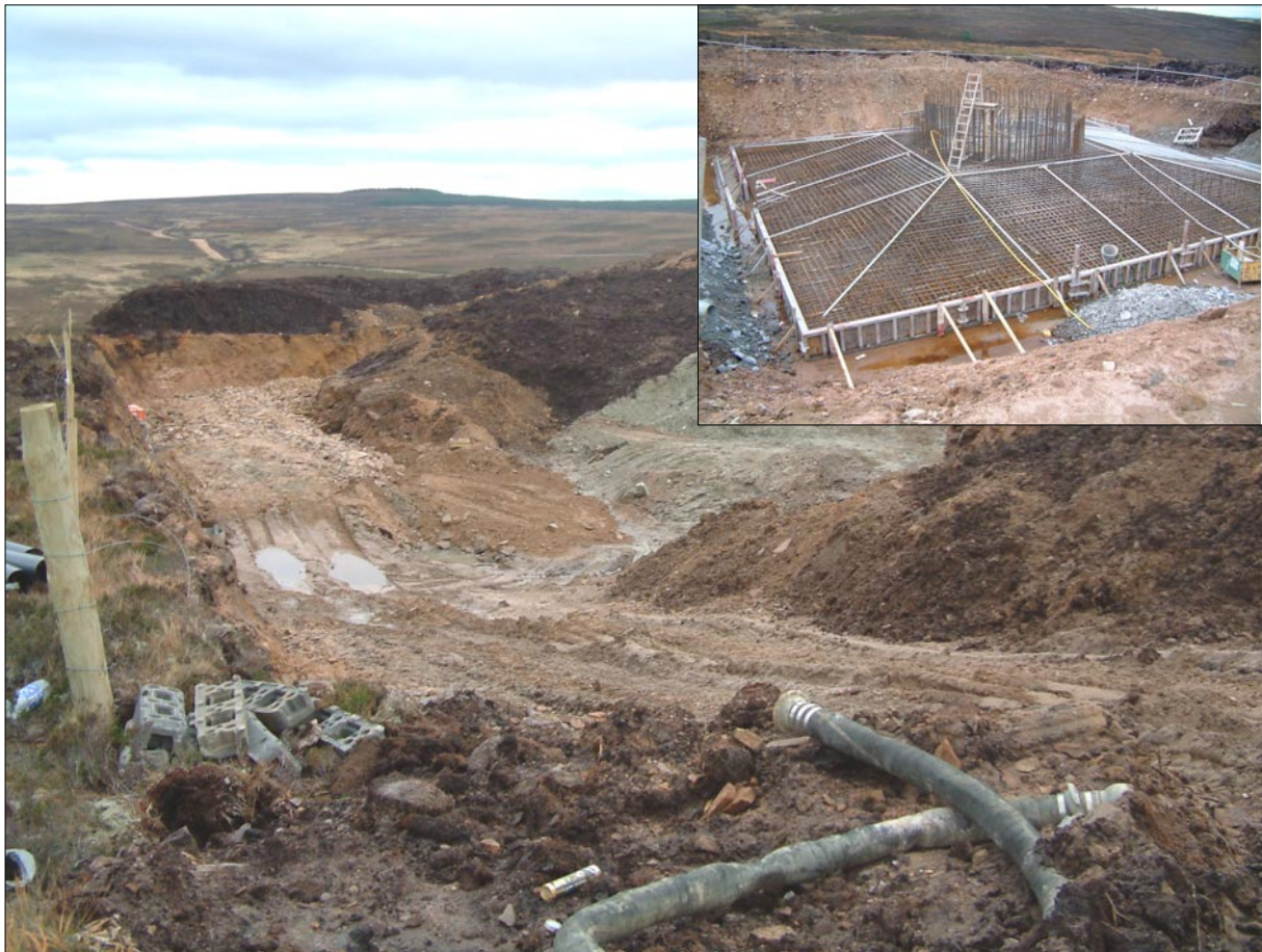
One of the smaller borrow-pits from the 28-turbine Cairn Uish site near Elgin and (inset) a turbine base nearing completion at the same site
