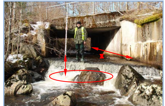
The Polmaily road culvert is a complete barrier to fish and needs to be modified to improve access for fish.
